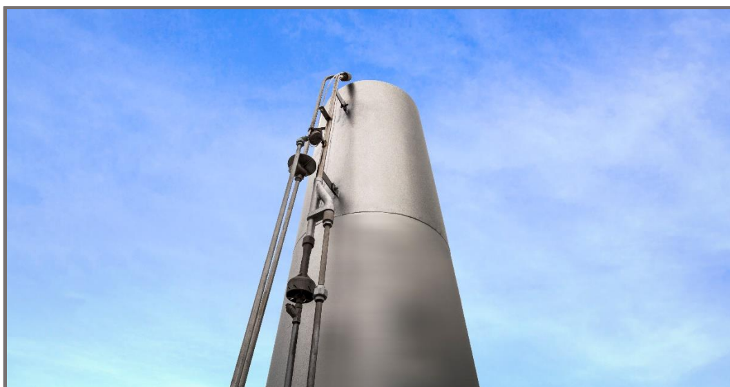
Figure 6: Fiber optic capable pilot on flare tip installation
